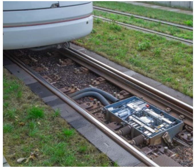
Point machine HW(E) 61.1 in the rail network
